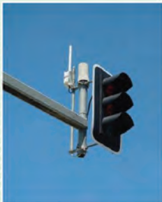
A traffic signal connected to a TMC using wireless communications technology
